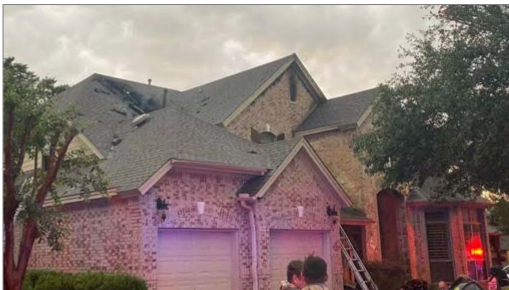
Figure 12-2. Damaged Home Resulting from Lightning Strike, April 28, 2023 4
